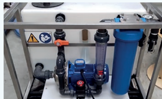
Chemical cleaning skid
